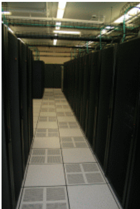
One of the server rack rows
