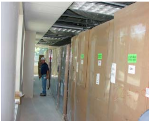
New equipment racks ready to be moved into the new facility.
