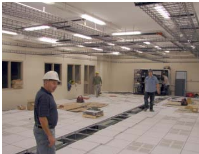
Looking east towards the Operations window from the west entrance to the Data Centre
